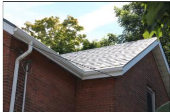
Composite roof materials may be an appropriate replacement material.
